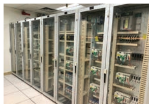
PLCs (Programmable Logic Controllers)
